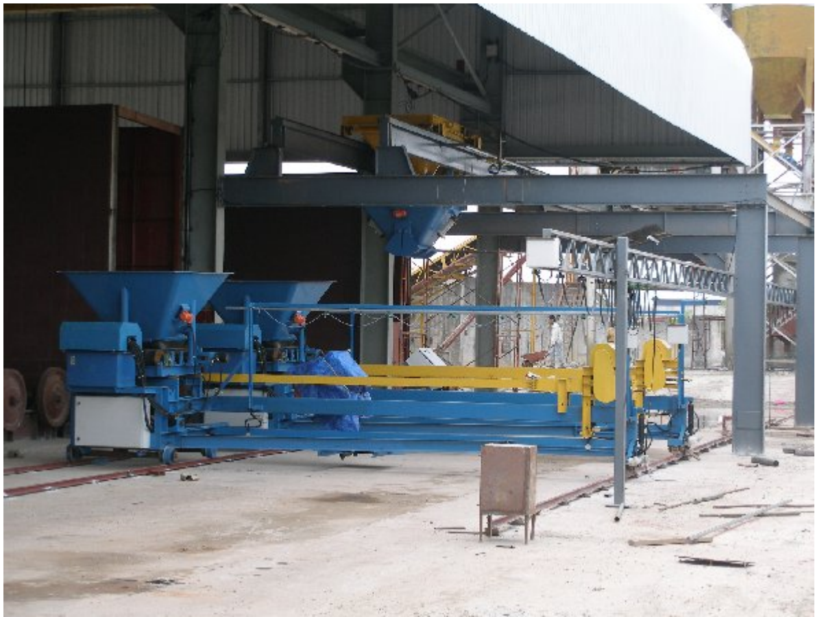
Spun Pipe Feeder Machine
